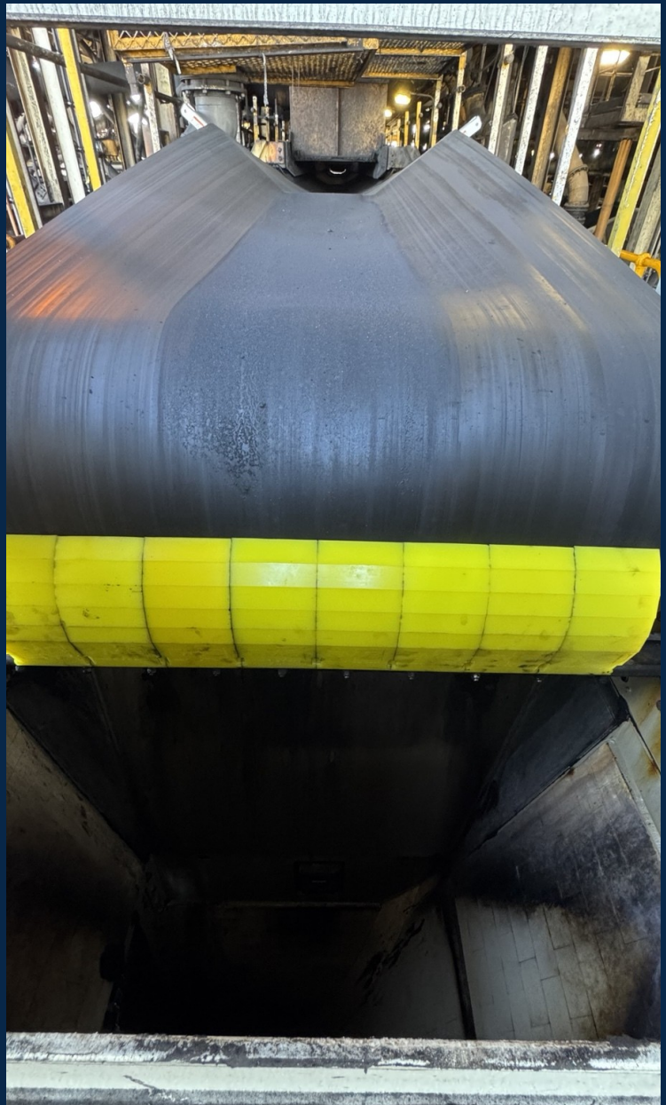
Yellow Super XHD primary cleaner installed in the head chute.
