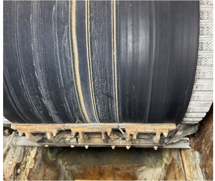
Longitudinal belt-cover damage at an old primary cleaner.
