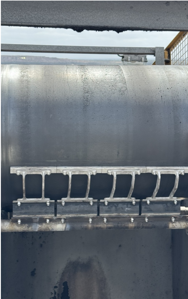
Primary Head Cleaner installed across the belt in the head chute.
