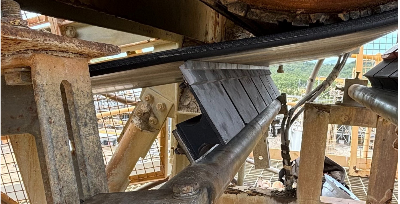
Single Direction Secondary beneath the head pulley, with the tip row, cushions and support pole visible.
