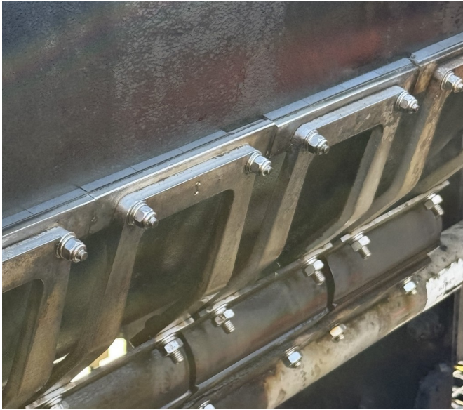
Dislodged Primary Head Cleaner tip segment disrupting the intended cleaning line.
