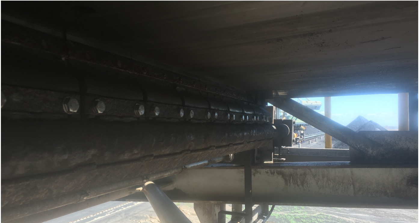
Reversible secondary cleaner installed beneath the belt, with the tip row and pole visible.
